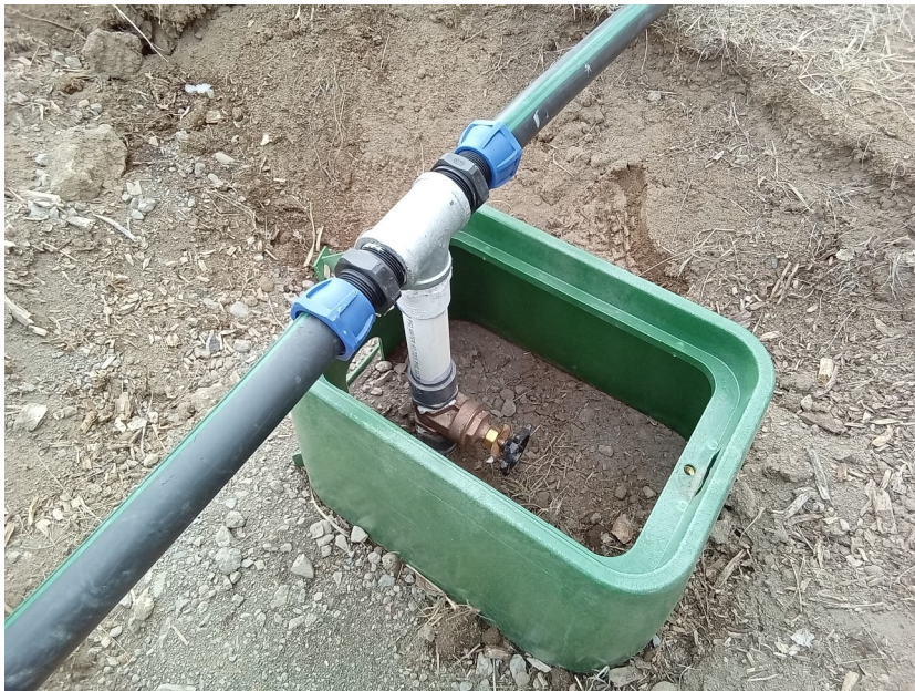
Typical Pod 2 line valve box
