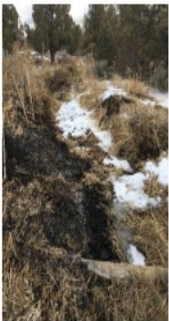
Before: Turnout from COID main canal. Broken headgate promoted sediment build up overflowing irrigation water to neighboring field and threatening well heads.
